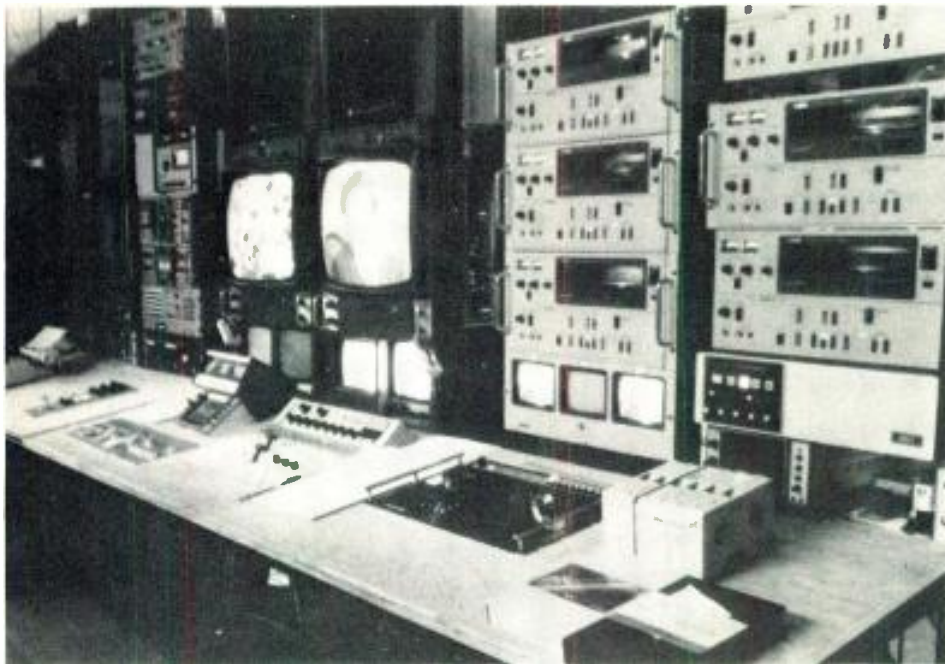
In master control, six U-Matics under microprocessor control provide majority of on-air signal.
