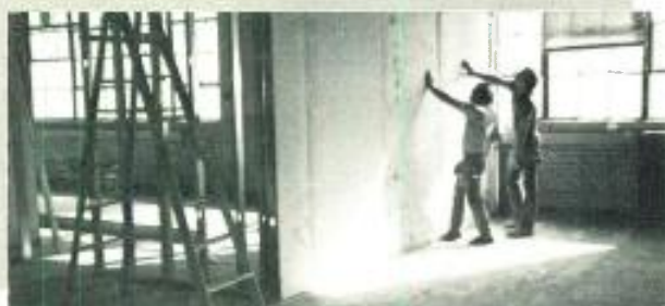
Workers install wallboard in offices that surround central working areas and studios.
